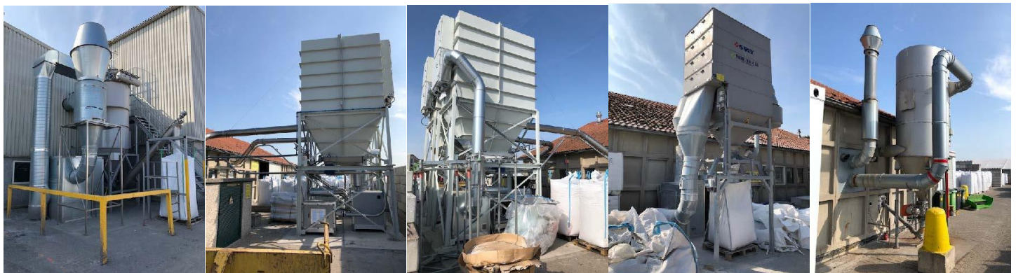
Figure 34 Air extraction and air cleaning systems of Plant D.
