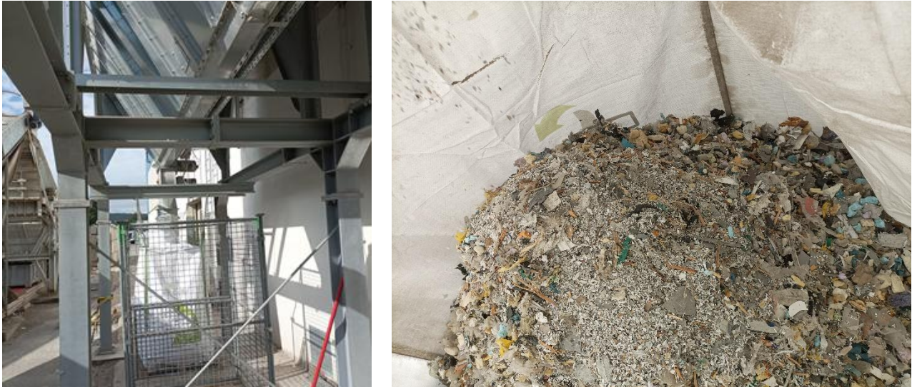
Figure 14 Air Extraction and filtering system. Left: the bottom view of the air extraction system with the big bag collecting the material removed from the air stream. Right: the inside of the big bag showing the dust and foamed or otherwise light material.
