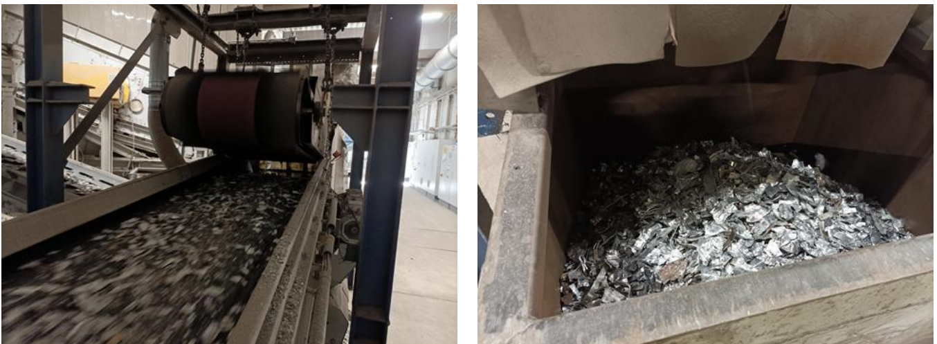
Figure 15 Magnetic sorting of shred profile waste. Left: shred material stream passing over magnet to remove ferrous metals. Right: separated ferrous metal.
