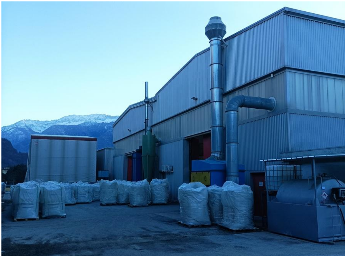
Figure 13 Channelled air emission systems Plant E. Extraction system to the left is equipped with a dust envelope filtering system. The extraction system to the right is equipped with carbon filters.
