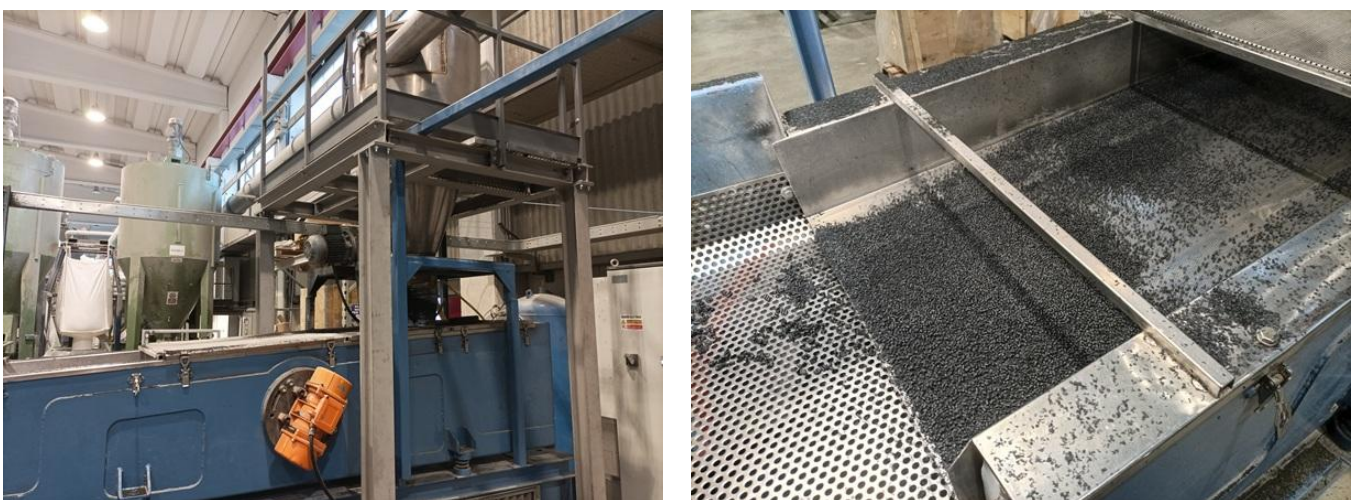
Figure 10 Pellet cooling station. Left: the first part of the cooling station where the material arrives pneumatically in the piping to a cyclone that then drops the pellets into the station. Right: the cooling station table where pellets are agitated and exchange their heat with an air stream.
