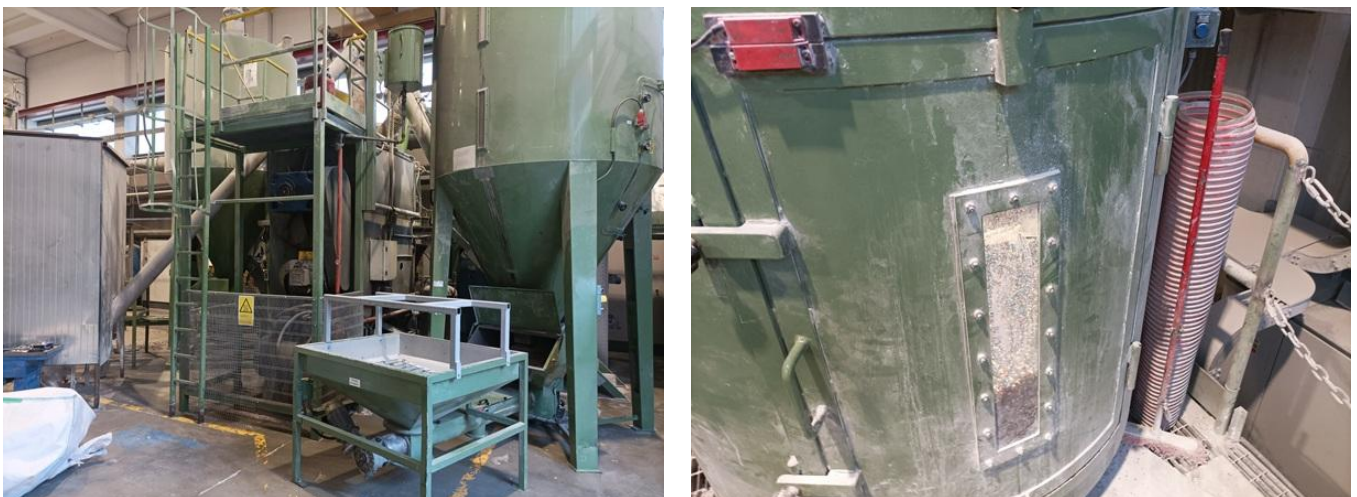
Figure 6 Silo for regrind prior to compounding and extrusion with melt filtration. Left: hopper feeding station. Right: silo with sight glass showing two different types of regrind flexible PVC.
